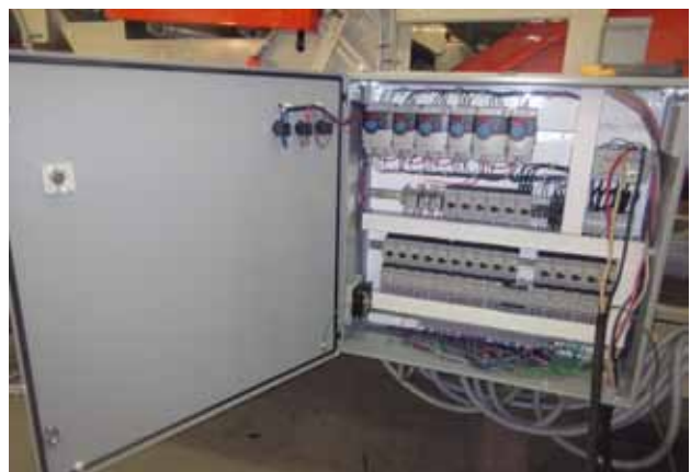
Variable Frequency Drive (VFD)
