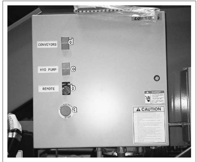
Fig. 3 MASTER CONTROL PANEL
